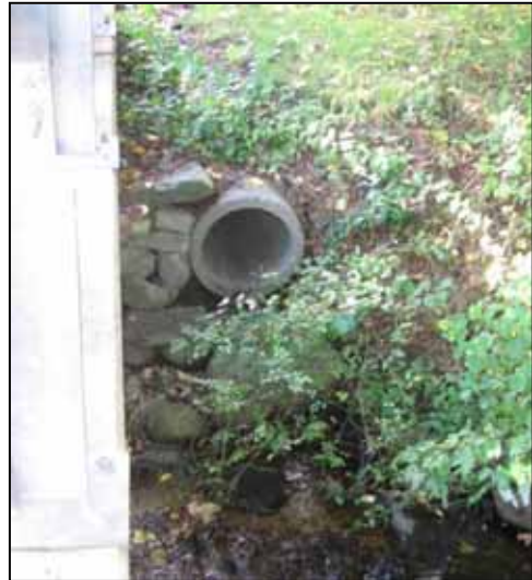
Stormwater outfall located in Peace Dale near Kingstown Road.
