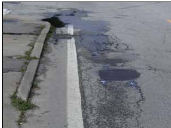
Paving conditions on High Street are in need of immediate repair.
