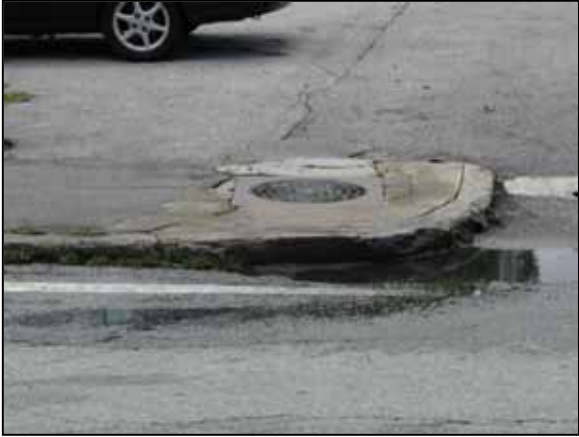
Drainage system on High Street can become overwhelmed during minor to moderate rain.
