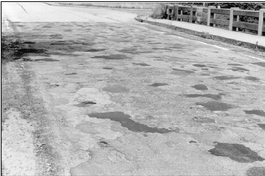
Shannock Road is in poor condition.
